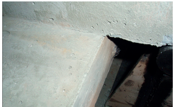
Fig. 6. Crack along the span at the junction of the
